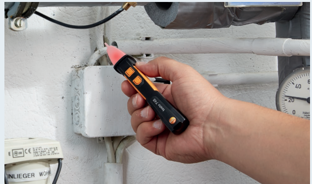
Non-contact voltage testing on a distributor box for a heating system with the testo 745.
